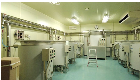
Thermal tank in the basic mash room
